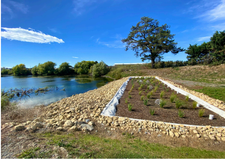
Lowes Pit Filterra® Bioscape®
